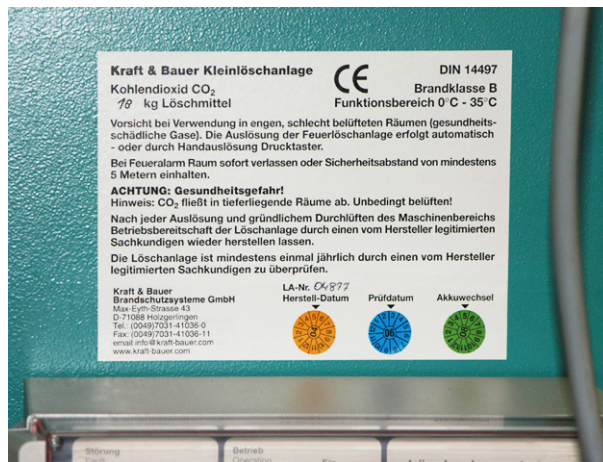
Example: Inspection stickers Kraft & Bauer
