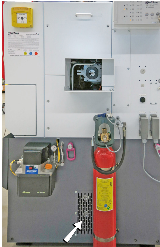
Fan in control cabinet TNL12.2
